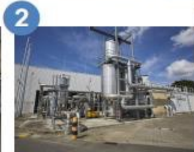
Biogas treatment plant
