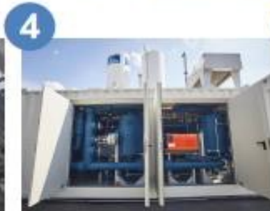
Liquefier and e-LNG filling Station
